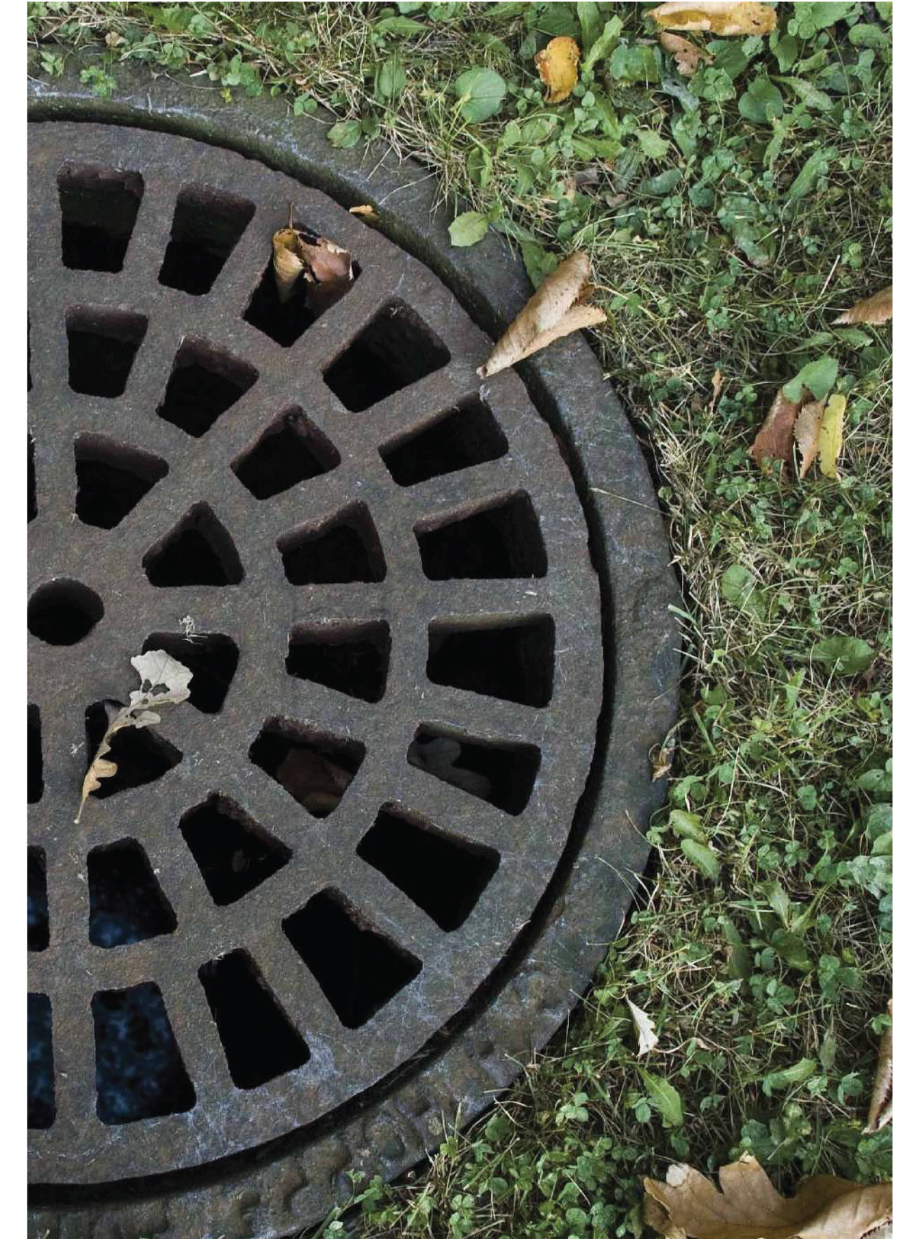
Storm Water Drains
