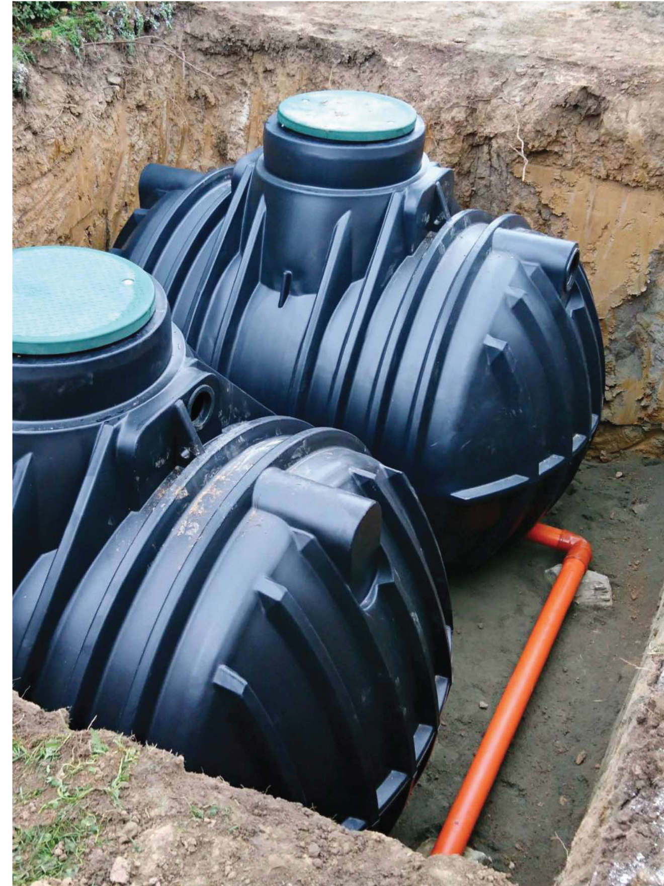
Rain Water Harvesting
